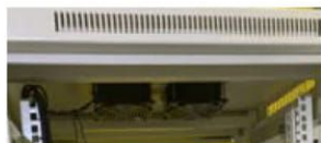
Fan units for dissipate heat
